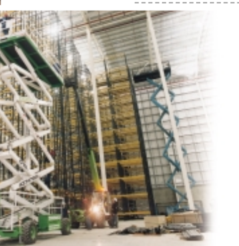
Link 51 installation teams use specialist skills, equipment and techniques to ensure racking is assembled safely and efficiently.
